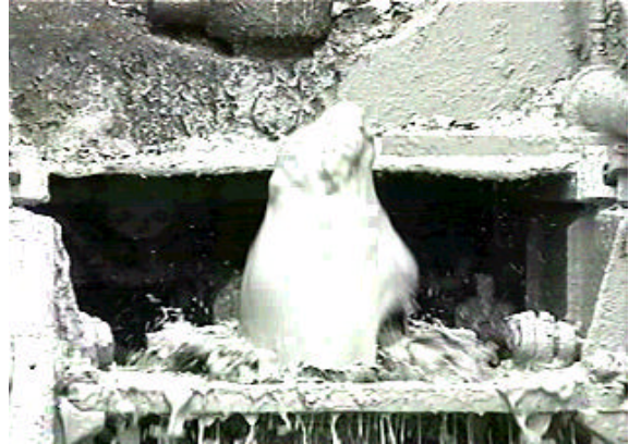
Tempest Environmental Systems drills through alternating layers of clay and quicksand to reach the underlying brackish aquifer.
